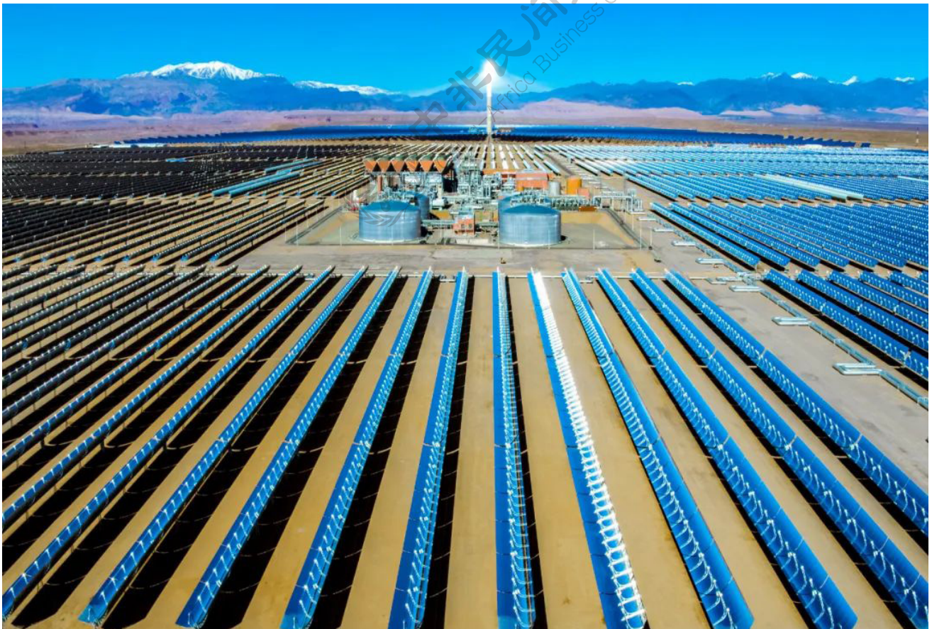
Figure 13 Noor III tower solar thermal power plant in Morocco
